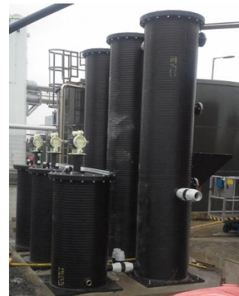
Figure 1 - CrumRubber Pilot Plant
