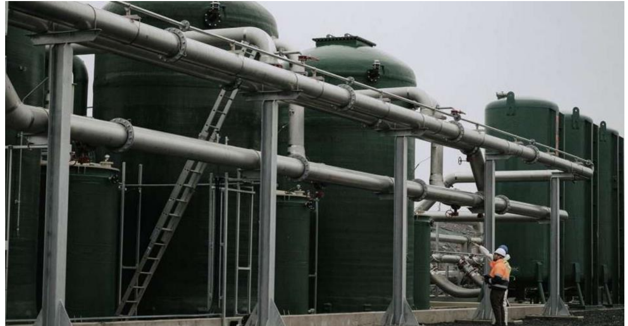
Figure 6 - CrumRubber Biogas Cleaning Plant
