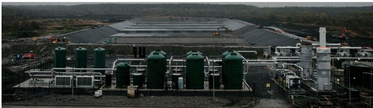
Figure 2 - CrumRubber Biogas Plant installed as part of a 5MW Landfill Gas Utilisation Plant at Drehid Landfill, Ireland
