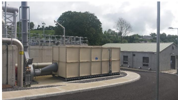
Figure 1 - Monashell OCU in Cavan WWTP, Ireland
